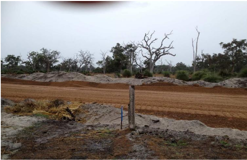
Photograph 4 – Location B looking North in proposed disturbance area in EmXp (existing Haul Road in foreground)
